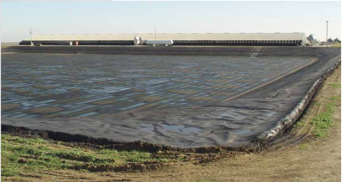
Figure 4. This floating impermeable cover was installed over an existing earthen manure storage lagoon.
